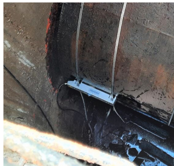
Clamp-on flow measurement of water in the spillway pipe
