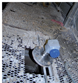
OPTIWAVE on gravel silo
