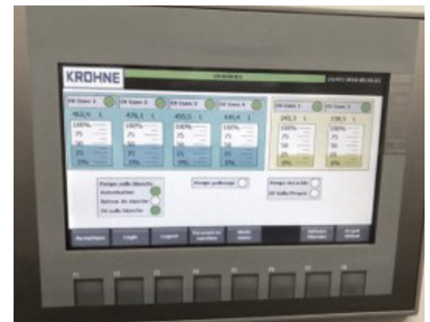
Level monitoring via the programmable logic controller (PLC)
