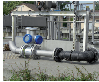
Test set-up at a sewage treatment plant
