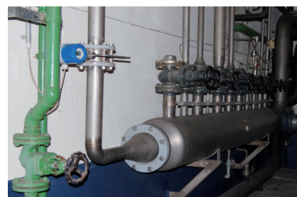
Distribution station for compressed air
