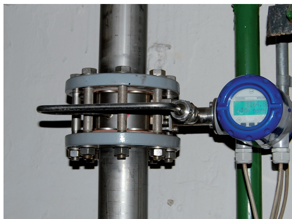
Constricted pipeline for flow measurement
