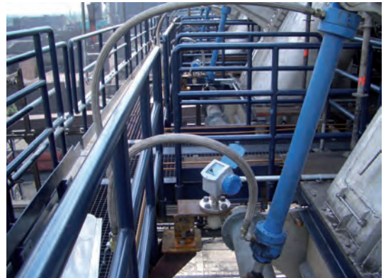
Four OPTIWAVE 6300 devices are installed next to the loading ramps
