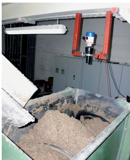
OPTISOUND 3010 above the mixing tank, one of the augers can be seen.
