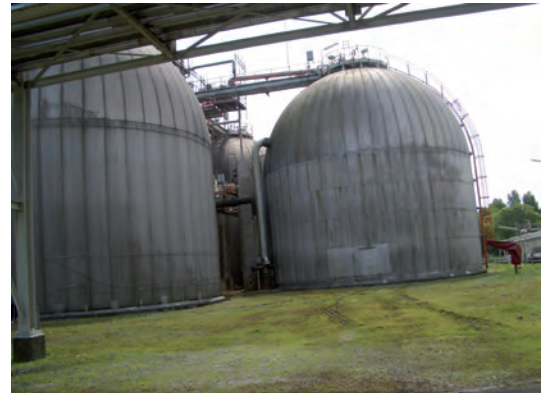
The spherical chlorine storage tanks may only be filled up to a predetermined height
