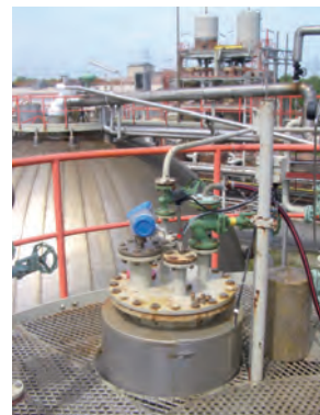
On the roof of the spherical tank: OPTIWAVE 7300 installed on the existing flange connectors
