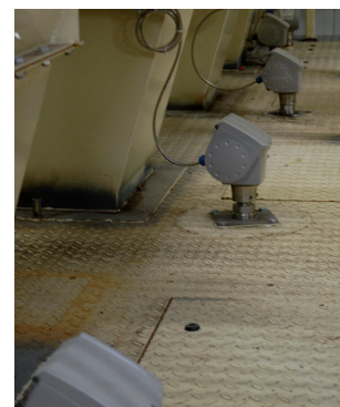
Installed devices on the silo roof
