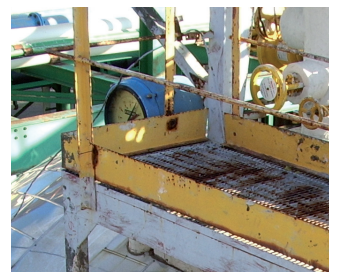
Old generation KROHNE BM 12 level meters
