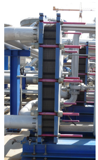
Cooling unit at calibration rig
