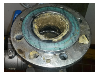
Pipeline from co-fermentation with large fat deposits
