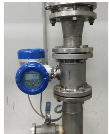
Flow measurement of fat for pump control
