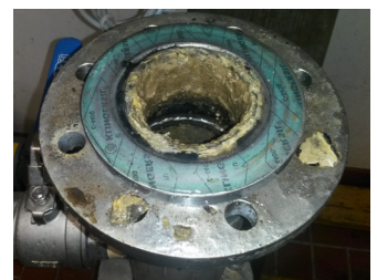
Pipeline from CO fermentation with large fat deposits
