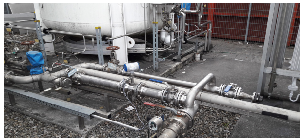
Nitrogen measurement behind built-in flow straightener
