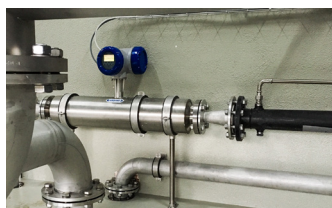
Measuring point with OPTIMASS 7400 C
