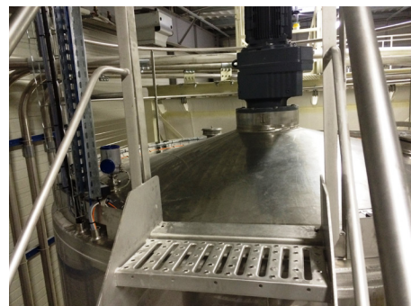
OPTIWAVE 3500 C installed on top of the tank
