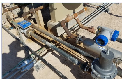
Allocation from wellsite through separator
