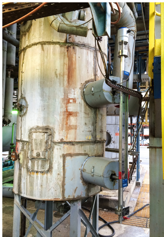
Bypass level measurement with the BM 26 W1010 connected to the steam condensate tank
