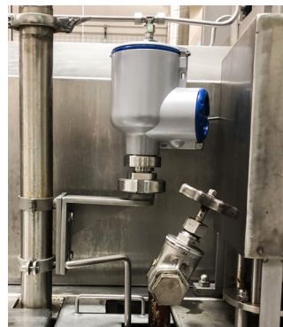
OPTIWAVE 3500 mounted above the tank of the deep fryer
