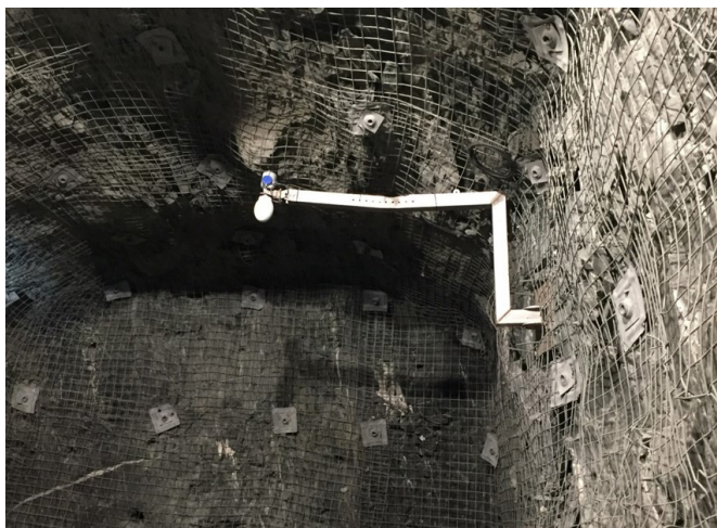
OPTIWAVE 6400 installed above ore pass
