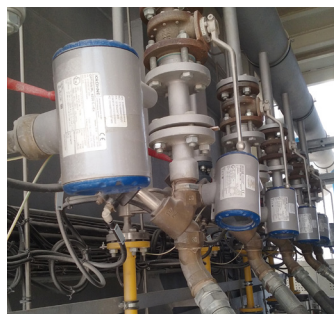
Vortex flowmeters installed into the supply lines to the gas burners
