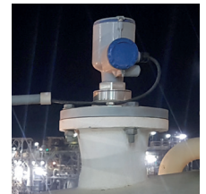
OPTIWAVE 7500 on ballast water tank
