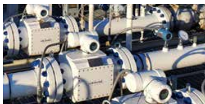
Gas fuel skids with ALTOSONIC V ultrasonic gas flowmeters
