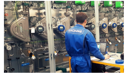
Combustion control cabinet with OPTIMASS 6400 Coriolis mass flowmeters for oxygen measurement
