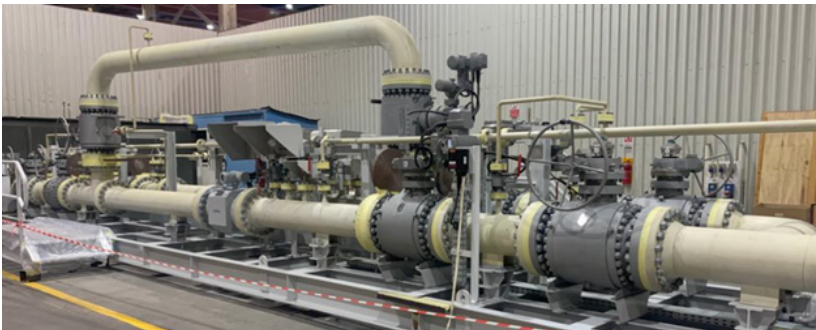
Dry gas metering skid with the ALTOSONIC V12 ultrasonic flowmeter
