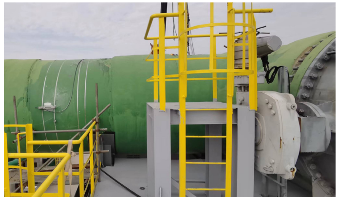
Installation of clamp-on flowmeter on large GRP pipe with reduced inlet and outlet runs
