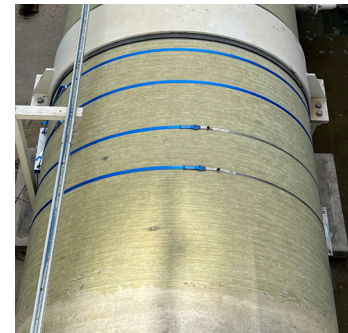
OPTISONIC 6300 P mounted with two rails on GRP pipe
