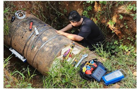
Commissioning of OPTISONIC 6300 P with two rails
