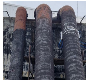
Clamp-on flow measurement on carbon steel pipe with bitumen coating
