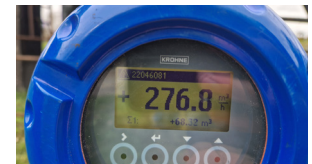
Wastewater flowrate displayed by Ultrasonic signal converter
