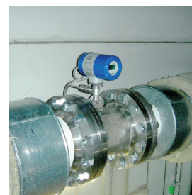
OPTISWIRL 4070 DN 200 at a measuring point directly behind a steam boiler
