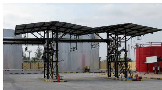
Filling station for 4 tankers
