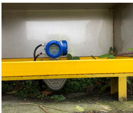
Measurement of the total hydrogen consumption with the OPTIMASS 6400 Coriolis mass flowmeter (DN15)
