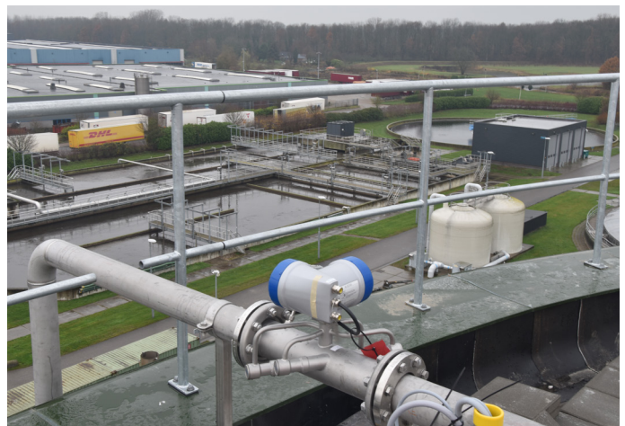
Flow measurement of biogas behind the digester
