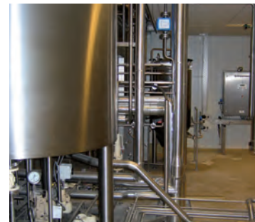
CO 2 recovery plant
