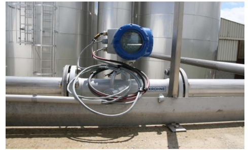
OPTISONIC 7300 Biogas in front of digestion tanks
