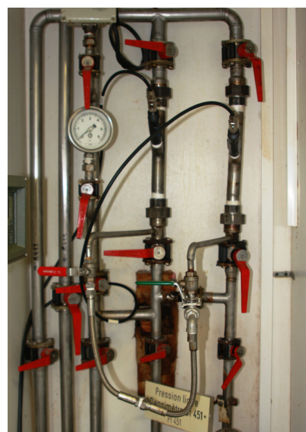
SMARTPAT PH 2390 installed between a hydrometer (left) and a redundant probe (right)
