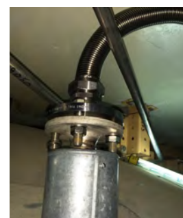
Transmission via coaxial cable with no electronics in the probe sub-assembly
