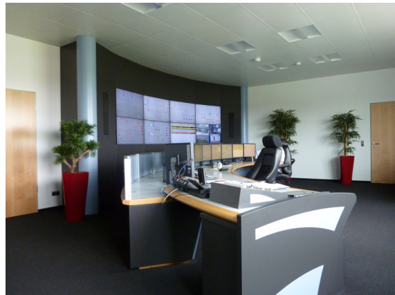
Leak detection in the control room
