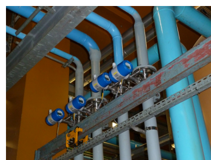
Vortex flowmeters measuring compressed air
