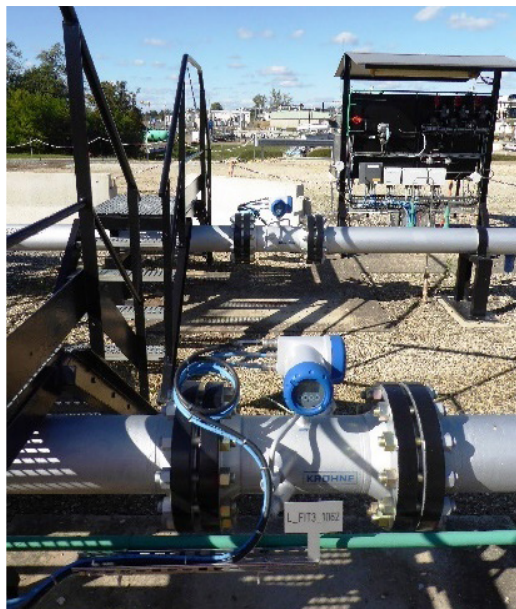
OPTISONIC 7300 ultrasonic flowmeter measuring natural gas
