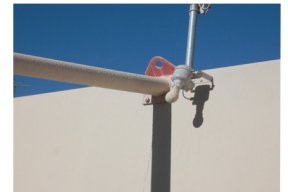
OPTIWAVE 6400 installed above feed hopper
