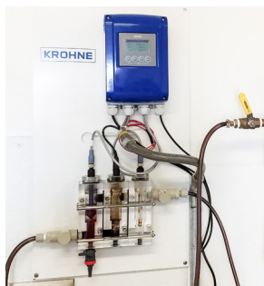
Installed OPTISYS CL 1100
