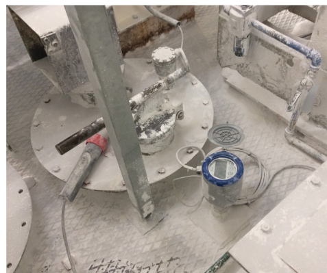
OPTIWAVE 6500 level transmitter on the storage silo
