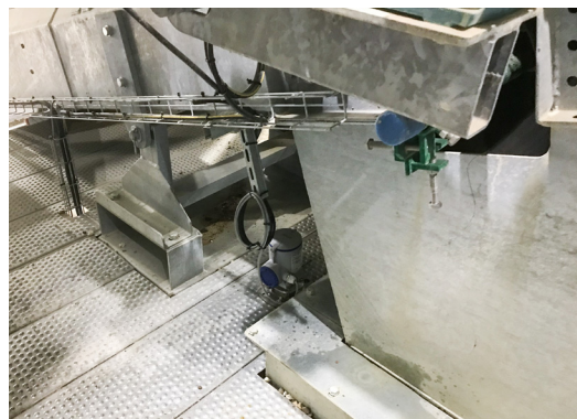
OPTIWAVE 6500 radar level transmitter on aggregate silo
