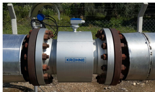
Ultrasonic flow measurement of geothermal brine
