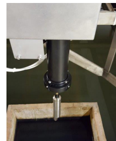
Sensor and cleaning unit of the sludge level measuring system
