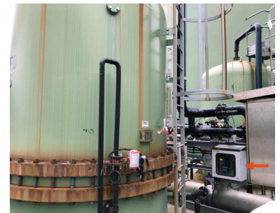
Air-conditioned control cabinet with KROHNE turbidity measuring system (see arrow)
