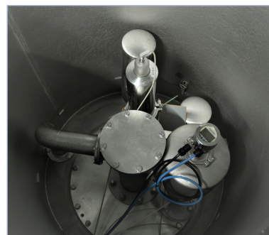
Installation of the primary pressure transmitter in a tank nozzle on top of the tank
