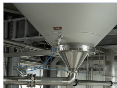
Installation of the secondary pressure transmitter at the conical tank bottom
