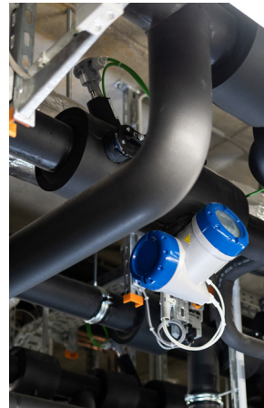
Electromagnetic flow measurement of hot water
