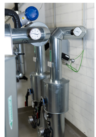
WATERFLUX 3300 measures the return flow to the geothermal probes
