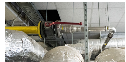
Natural gas pipeline with renewed, tapered piping on the right
