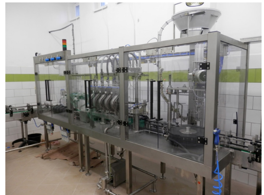
OPTIBATCH 4011 installed in parallel on the linear PET filling machine
